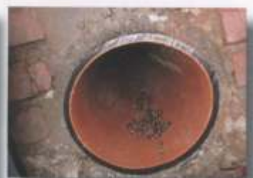
After applying the TIP technique, the new pipe lies tightly adjacent to the old pipe wall.
