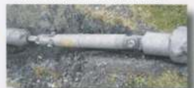
Grundolog III measuring unit for pulling force recording and log, mounted between backreamer and pipe puller.
